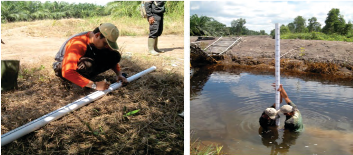
Gambar 5. Pemasangan water level pada intake/ inlet Sungai Antasan Mastam Figure 5. Installation of water level at the Antasan Mastam River intake / inlet
